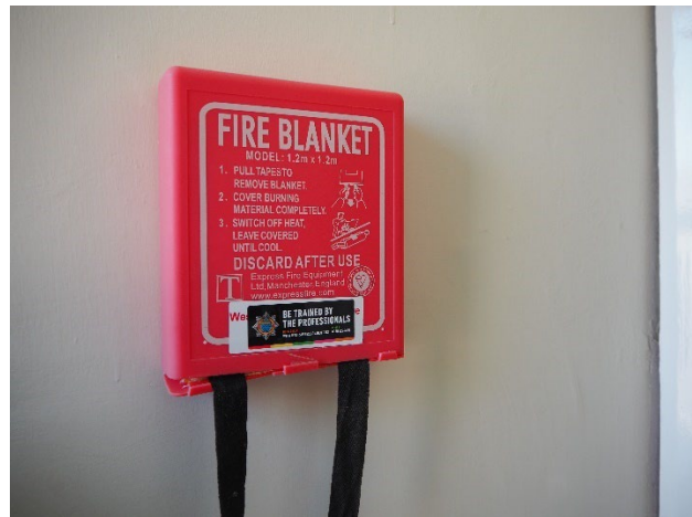
A Fire blanket is provided.
