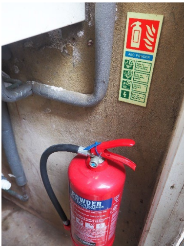
Boiler room, dry powder fire extinguisher.
