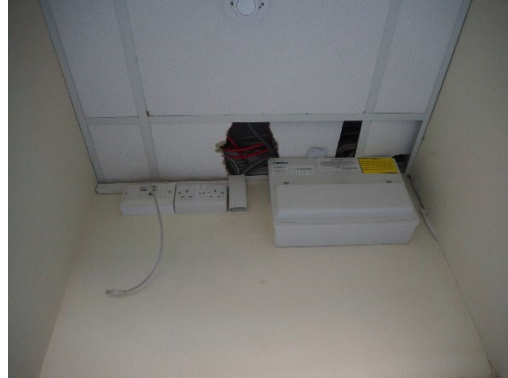
The ceiling tiles should be replaced to ensure integrity of fire stopping.
