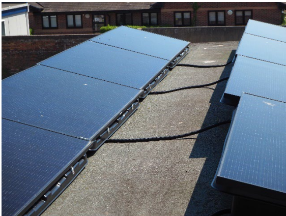
Solar panels are located on the roof of second floor at the rear of the building.
