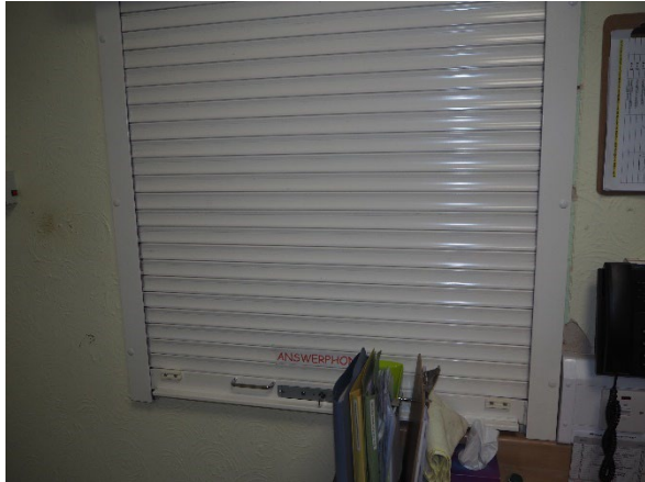
Inside view of fire roller shutter in down position.
